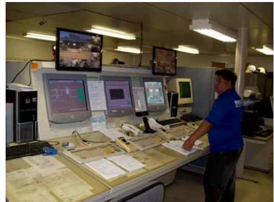
The engine control room of PB 117 where the monitoring of all machinery activities, performance, alarms and remote control operation is done.
