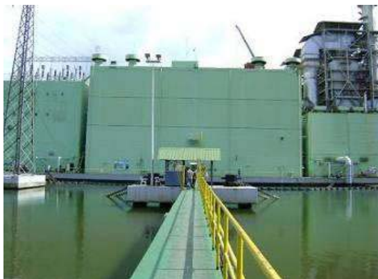
100-MW PB 118 located in Barangay San Roque, Maco Davao del Norte
