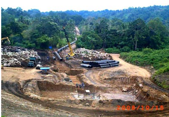
Reservoir A and Penstock
